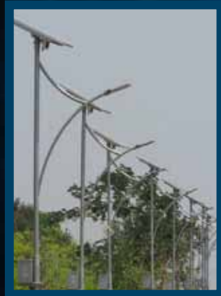
Solar Street Lighting
